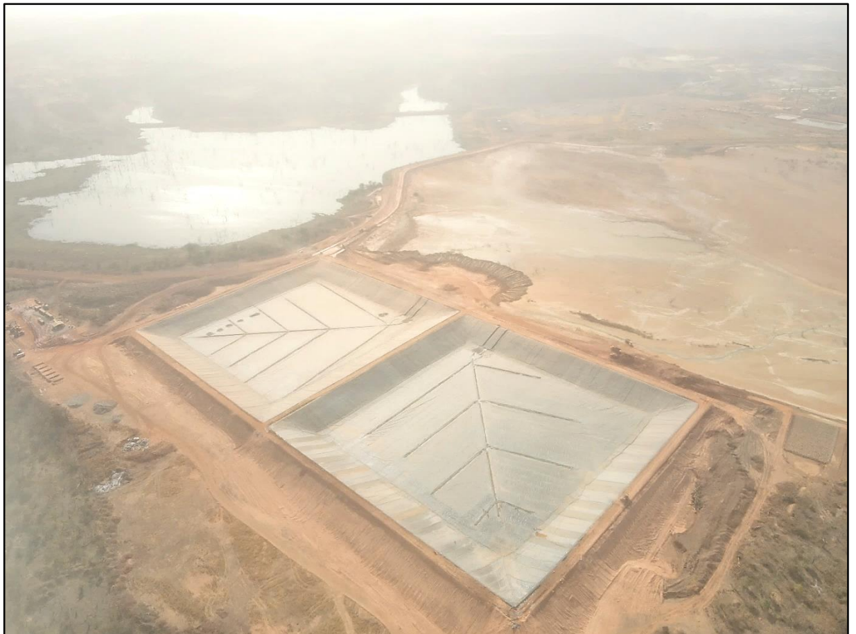
Figure 10: Tailings storage facility ("TSF") 1b comprising two HDPE lined cells has been completed
