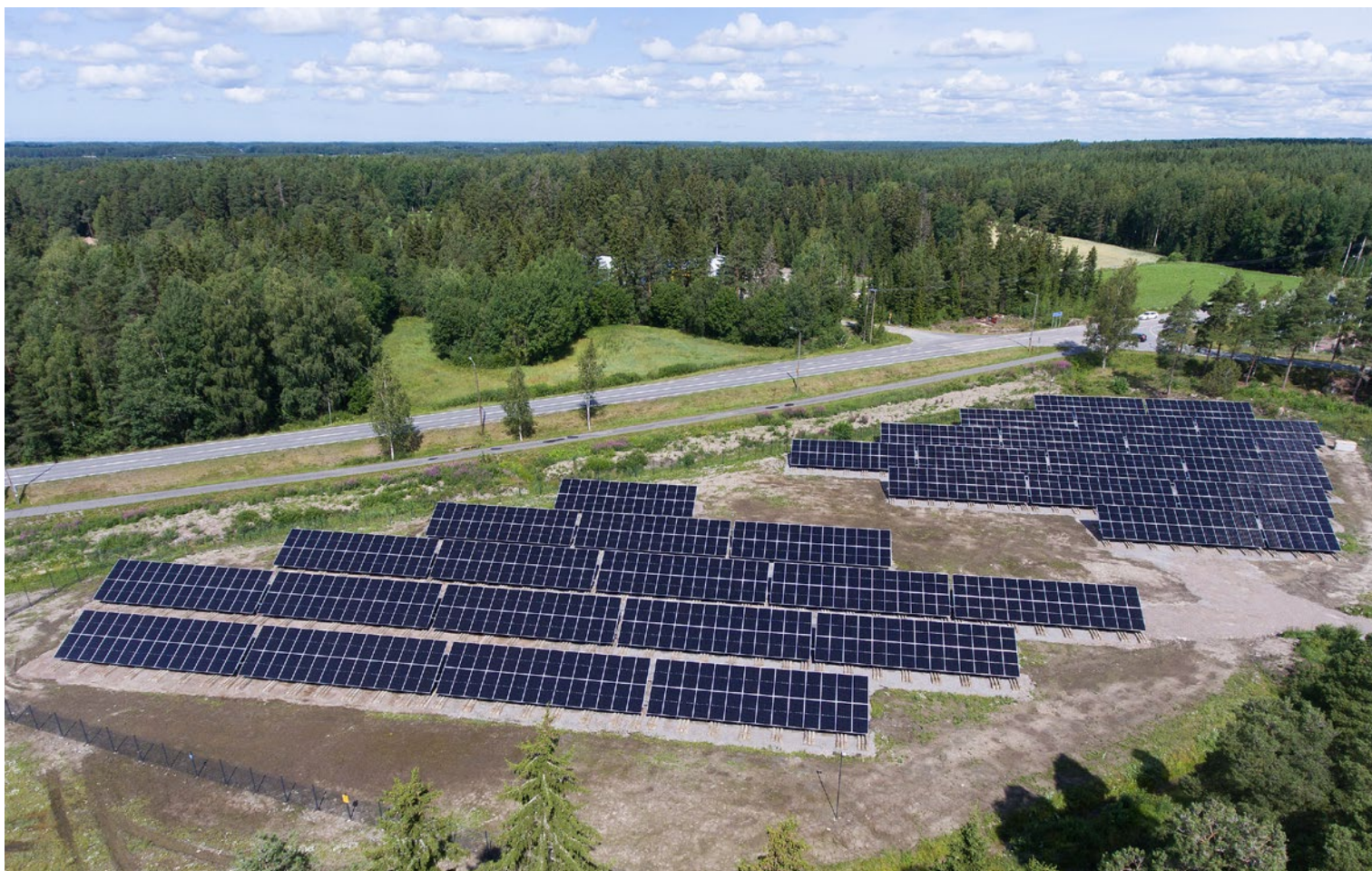
Solar park at Coreplast Laitila Oy.
