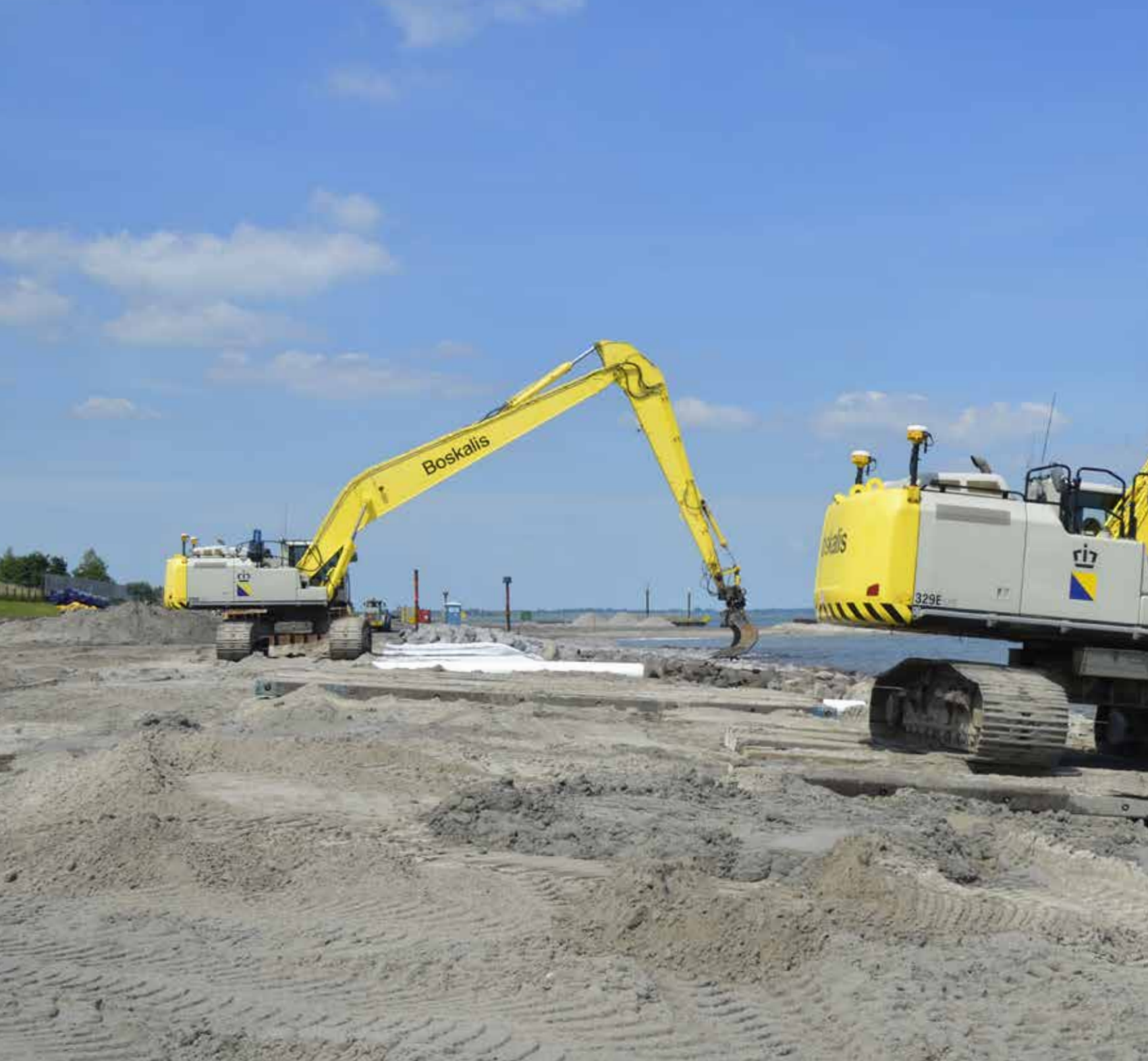
Earthmoving activities in connection with the reinforcement of the Markermeer dikes in the Netherlands
