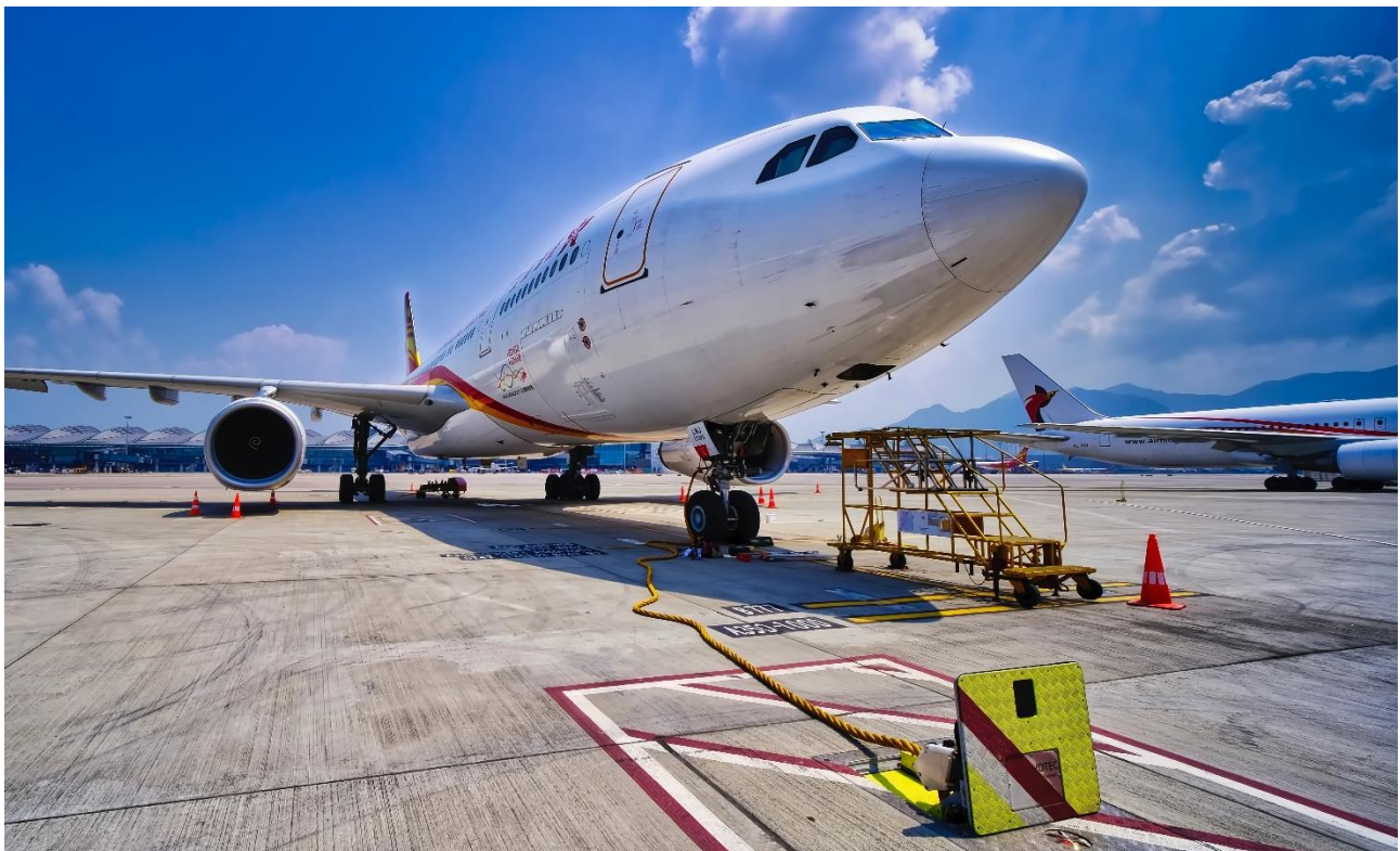
Cavotec Hatch Pit in-ground system supplying 400Hz power to an aircraft at Hong Kong International Airport.
