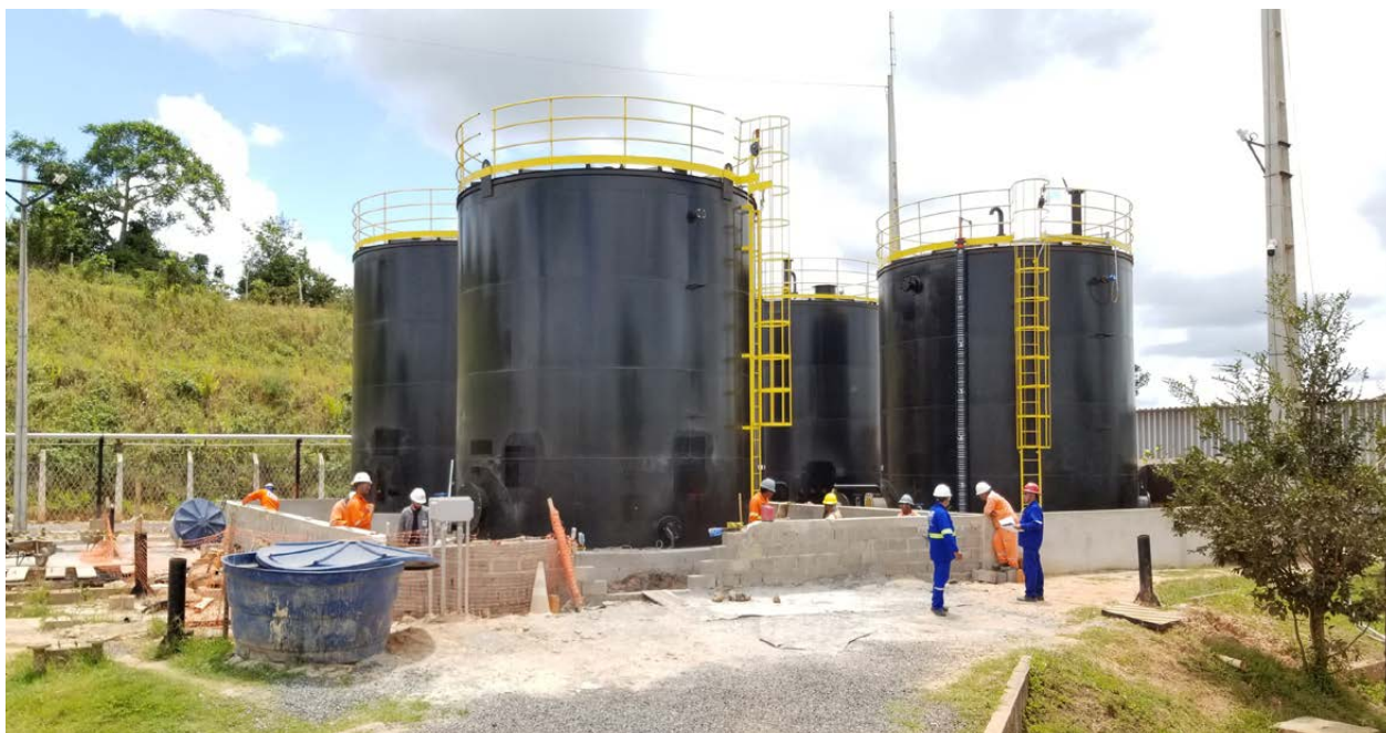
Four new 1,000 bbls oil storage tanks
