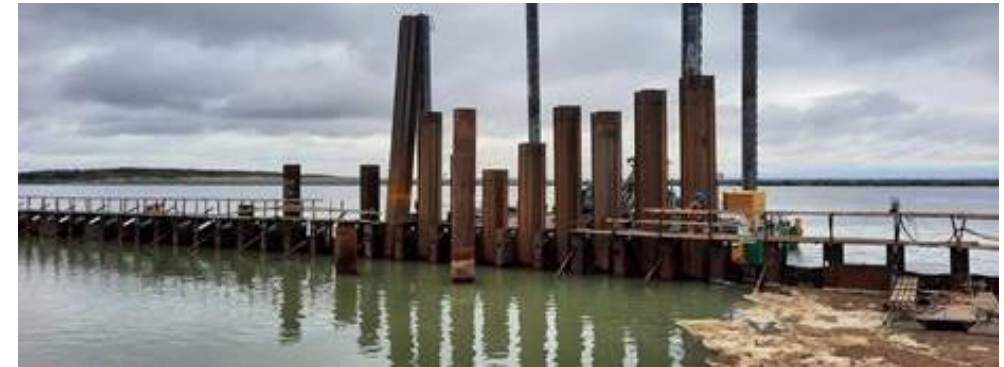
RECONSTRUCTION OF BERTHS. PHASE I. CONSTRUCTION OF NEW BERTH. INSTALLATION OF THE SUPRASTRUCTURE Construction works are underway, installation of berth load-bearing structures and engineering networks, technological pipelines
