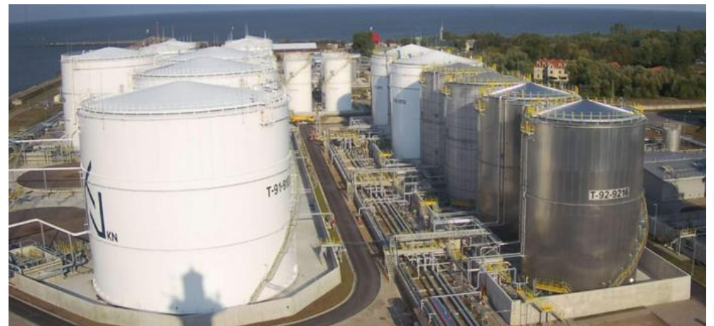
EXPANSION OF KLAIPĖDA OIL TERMINAL TANKS PARK Construction work is completed, final equipment tests and adjustments are underway.
