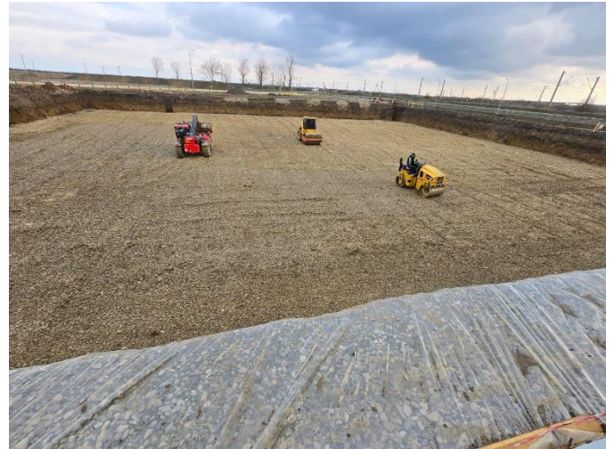
The preparatory work is on full speed. A four-meter-deep pit measuring 50 x 50 meters is excavated for the foundation to carry the four new silos, each capable of holding 6,000 tons.
