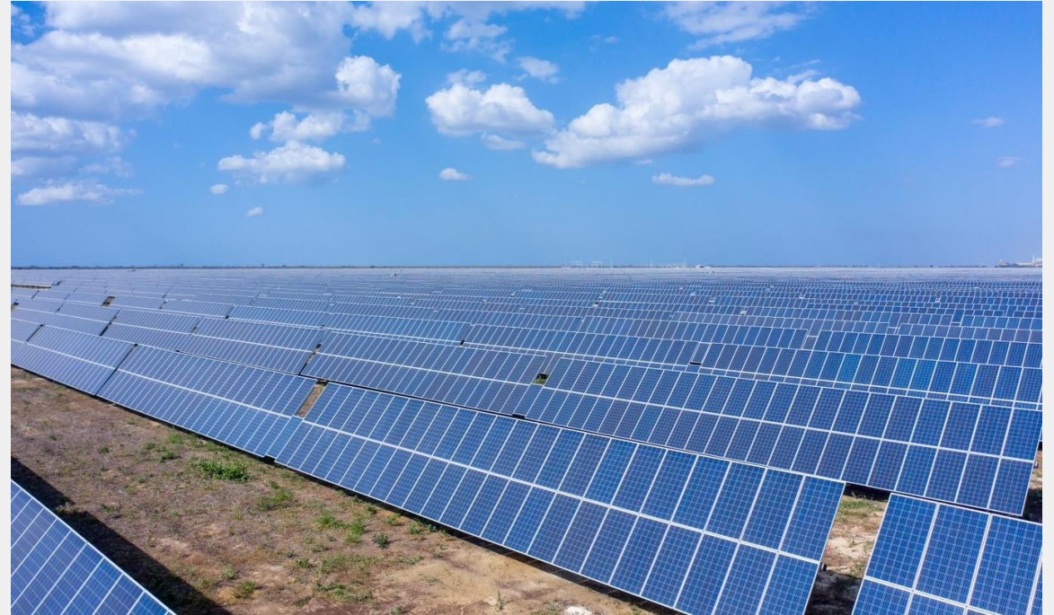
The 162 MW Apodi solar plant in Brazil.
