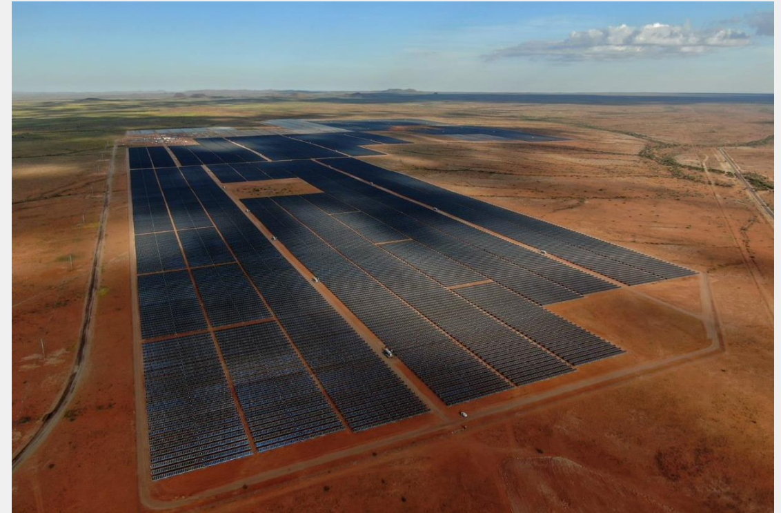
The 258 MW Uppington project in South Africa.
