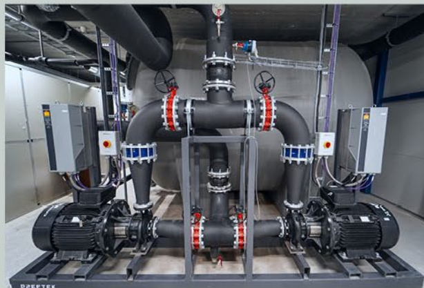
Picture of our new process water recycling plant
