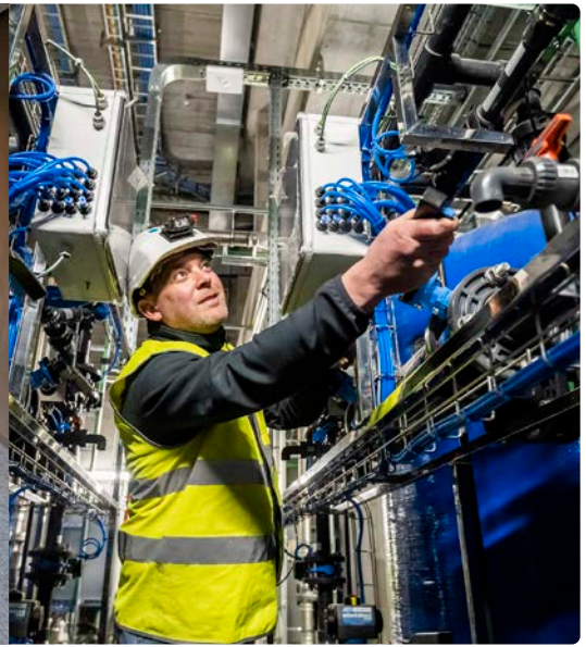
CFE • VMA (Multitechnics) at Grand Hôpital de Charleroi
