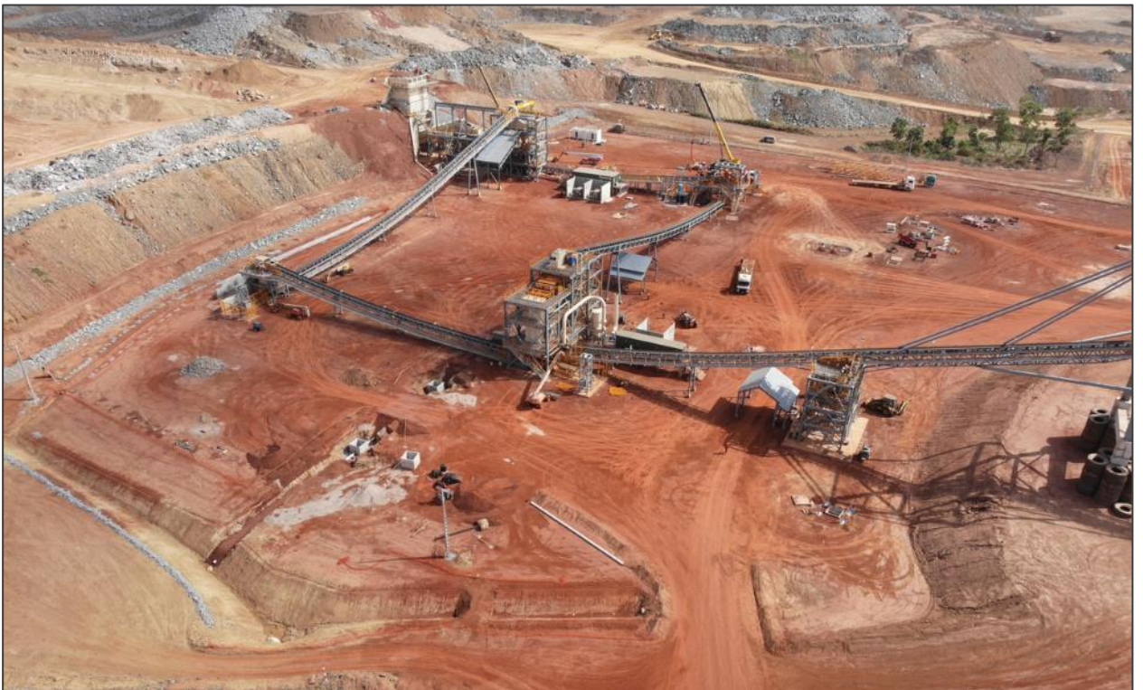
Figure 2: Primary crushing circuit with wet commissioning in progress
