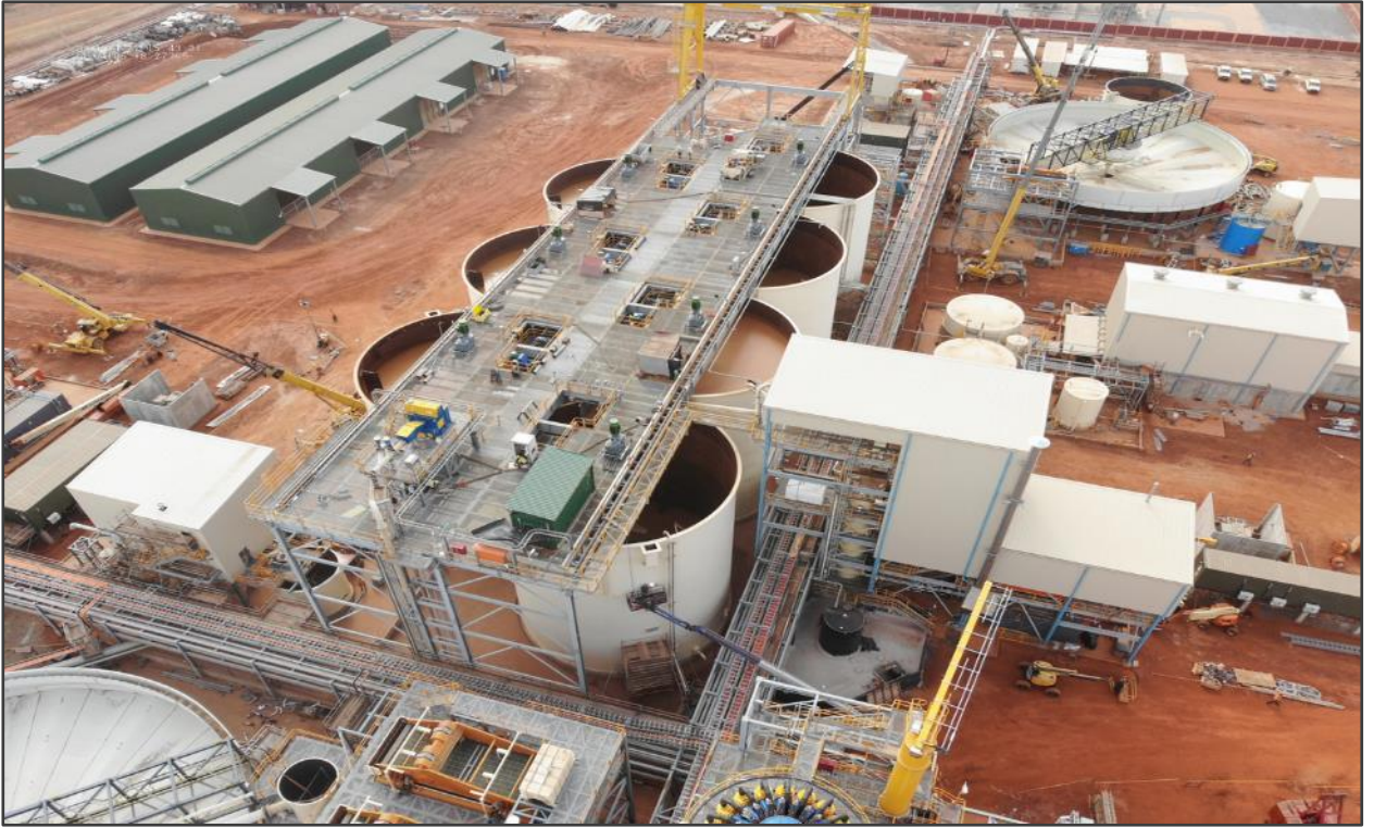
Figure 5: Wet commissioning of the CIL circuit is underway
