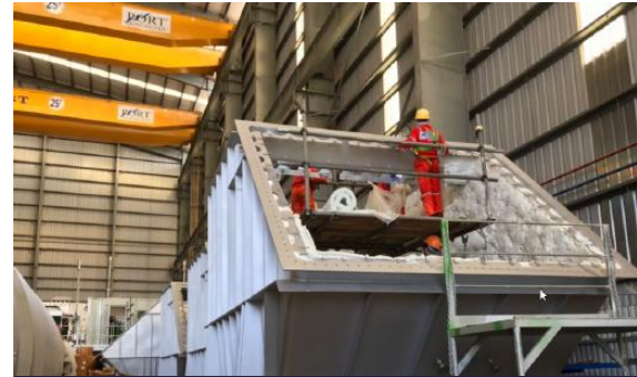
Y-Ducts for Heat Recovery Steam Generators (Kanfa)
