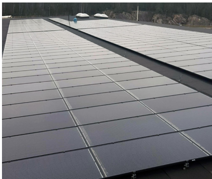
570 square metres of roof is being used to produce power.
