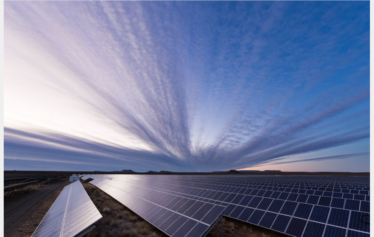
The 75 MW Kalkbult solar plant, South Africa.
