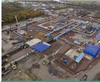
Nord Stream 2 onshore facility
