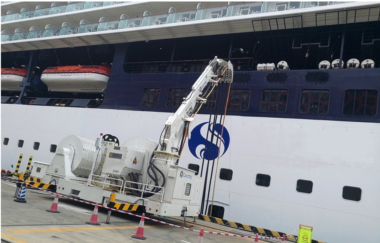
A battery-powered AMPMobile unit connects a ship to shore power at Shenzhen cruise terminal.
