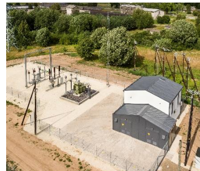
Estonia's leading builder of substations
