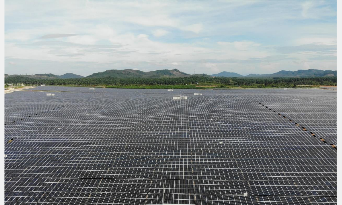
Gurun, part of the 197 MW Quantum Solar Park, Malaysia.
